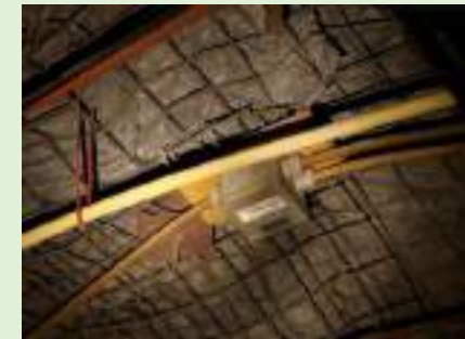
Voice communication infrastructure
